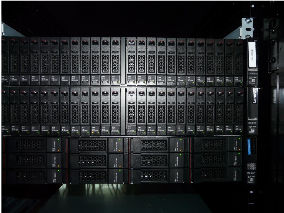
Photo 1. The appearance of Lenovo ThinkSystem DS2200 SFF FC/iSCSI Dual Controller Unit mounted into the server stand
